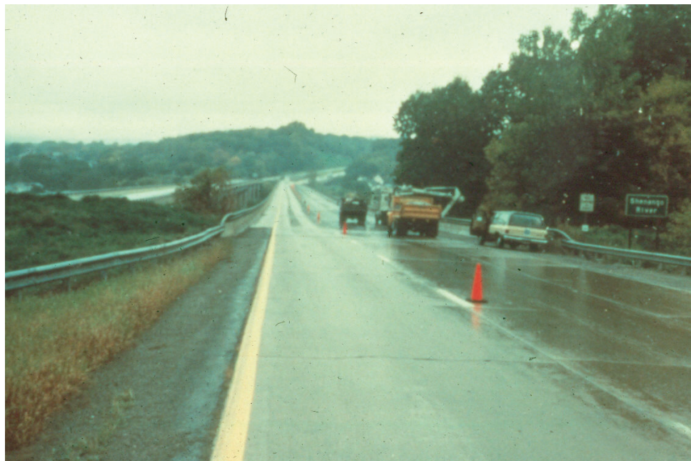
Figure 3.2.8 Inclement Weather Causing Slippery Bridge Members and Poor Visibility for Motorists
